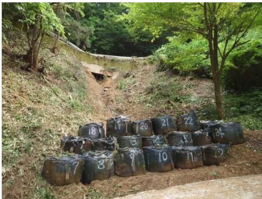
▲被災箇所①
